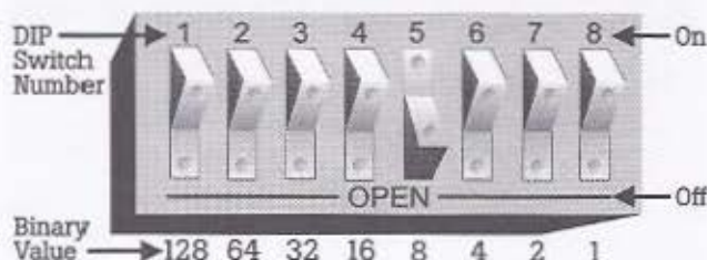
Figure 23 TUC DIP Switches set for Address 8
